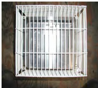
VIEW OF SAFETY CAGE
